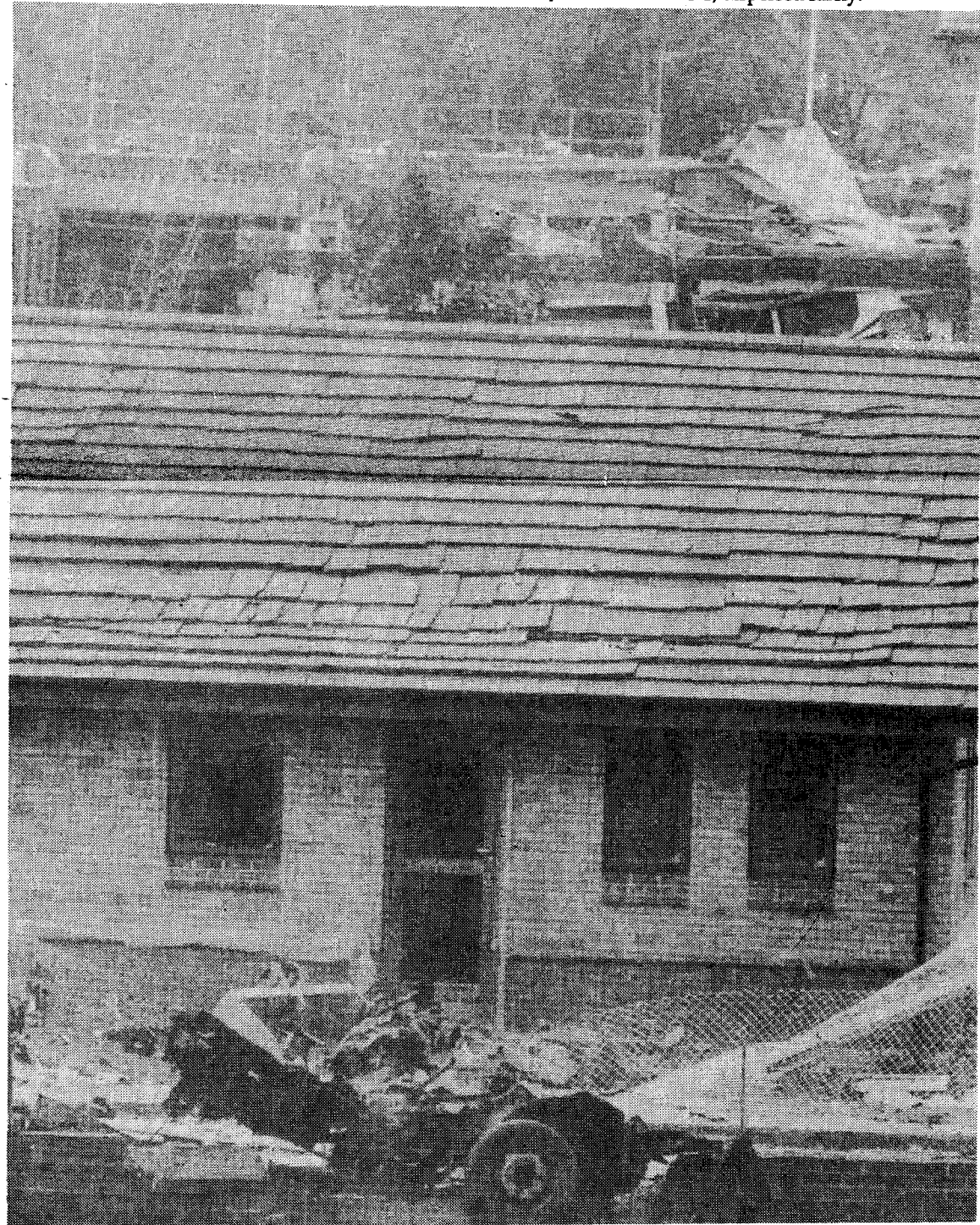
● Extensive structural damage was caused to the RIR's centre of operations in Belfast in a daring mortar attack by the Irish Republican Army
