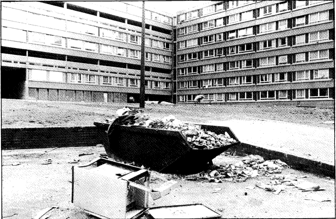
● The failure by the Housing Executive to provide adequate waste disposal facilities has led to some tenants having to burn their rubbish to stem the plague of rats which infests Divis
